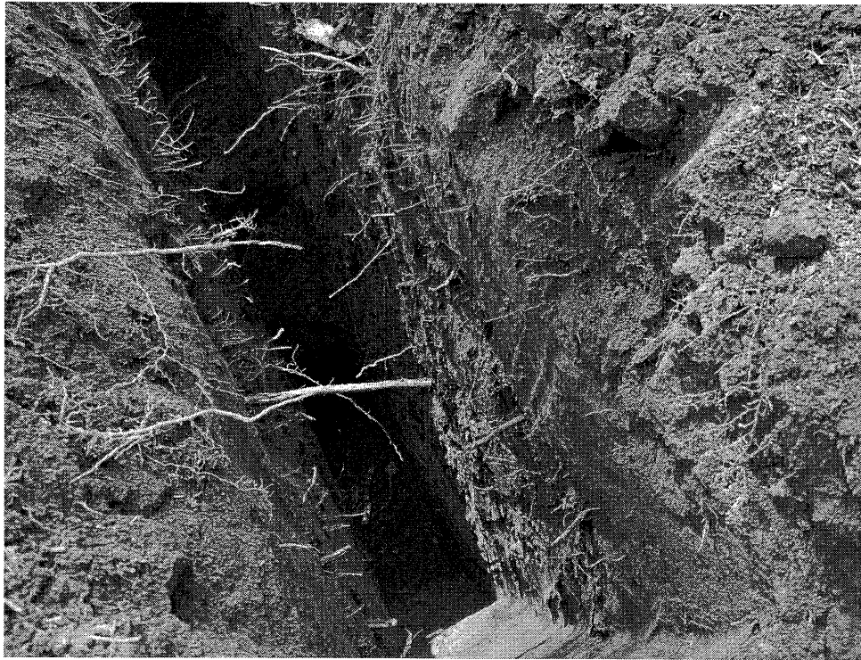
Photo No. 2 - Evidence of heavy root and forest duff within the upper two feet of TP1
