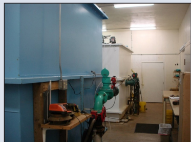
Old Water Treatment Units
