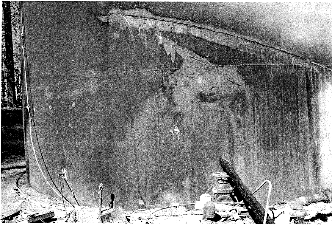
Damaged tank wall
