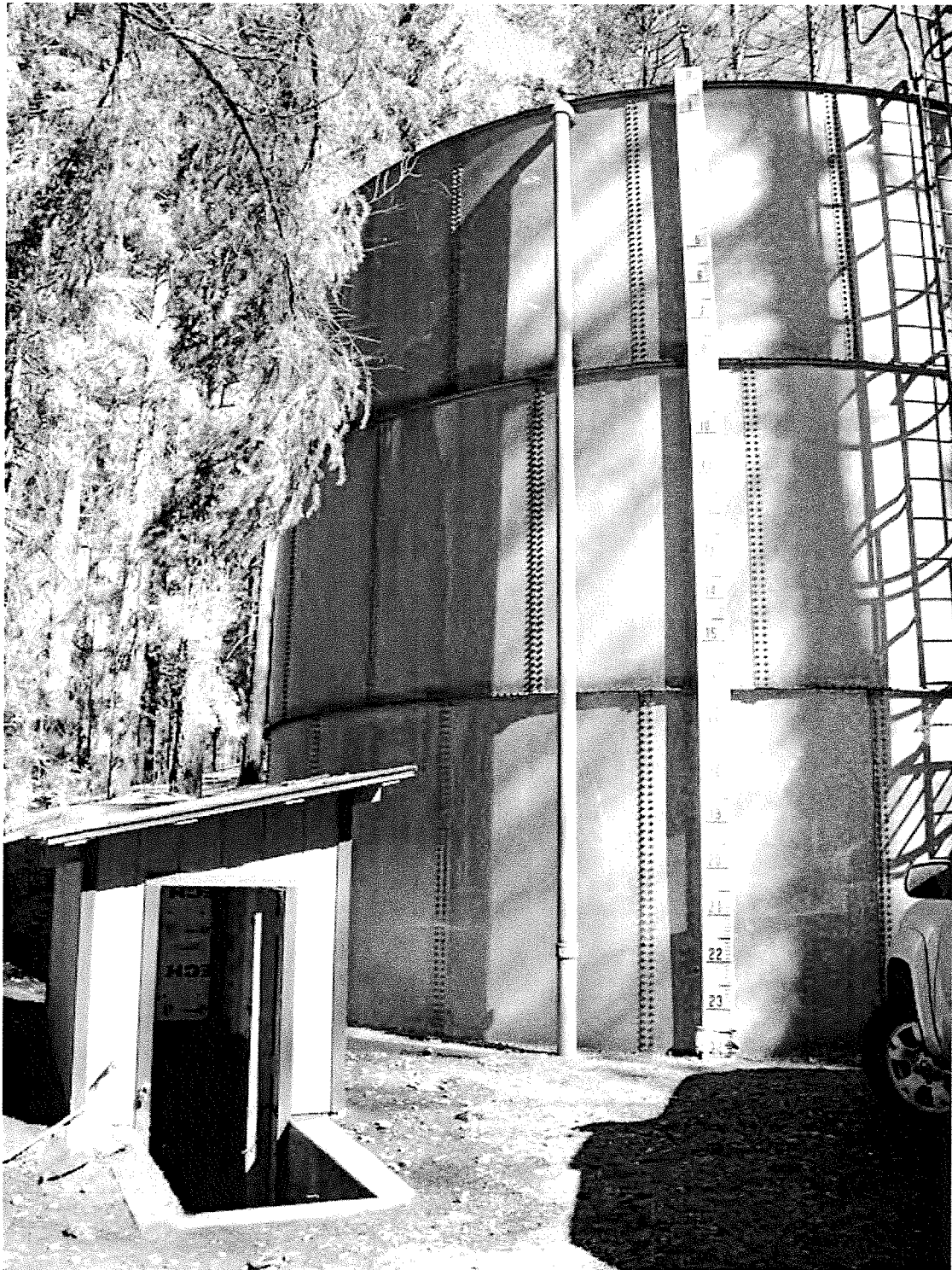
Winding Way bolted tank
