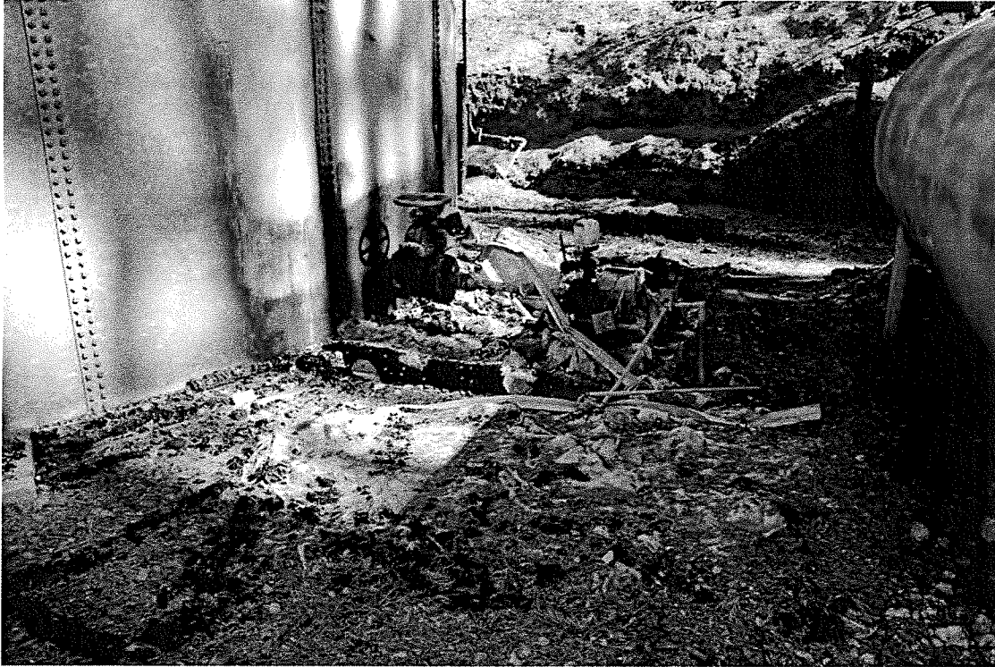
Destroyed equipment at tank outlet
