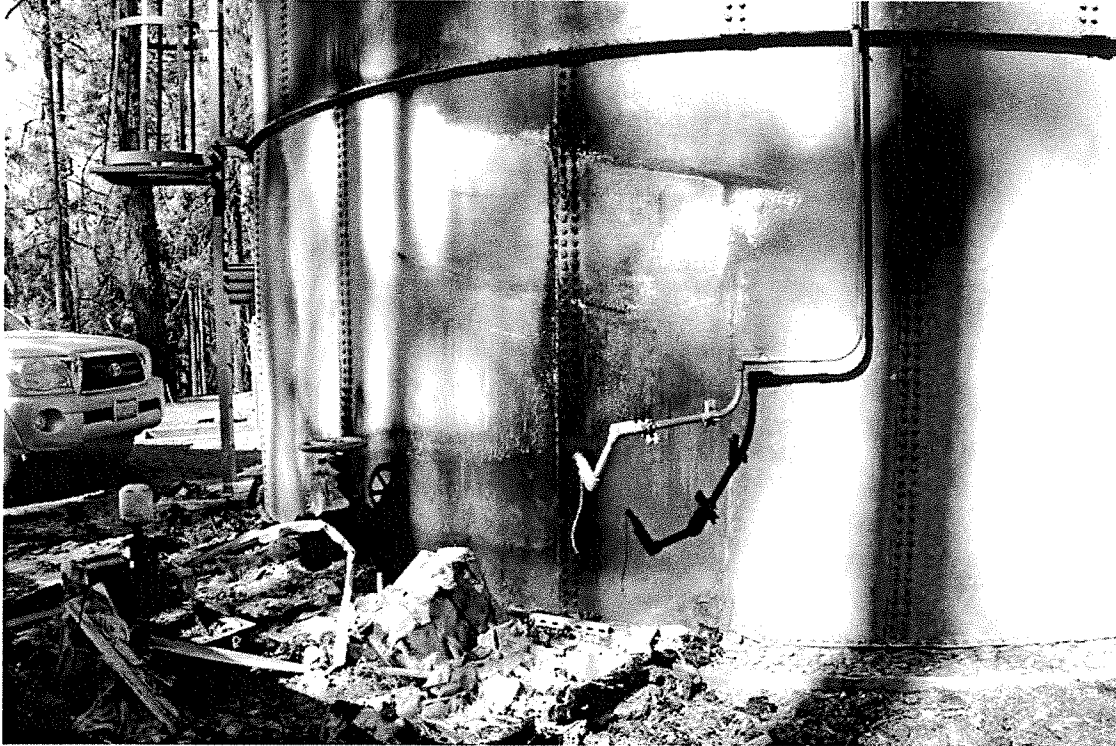
Damaged tank wall
